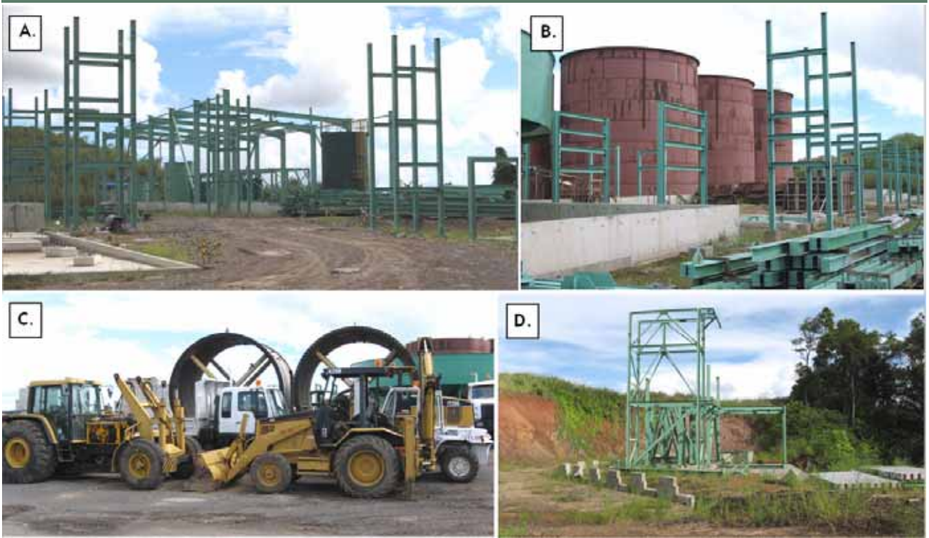
(A) Mill Framework, (B) Leach Tanks, (C) Ball Mill and Machinery, and (D) Steelwork for Rotary Crusher
